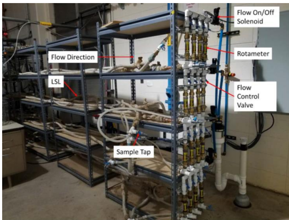
FIGURE 7: LEAD PIPE RACK AT THE MARSTON TREATMENT PLANT
